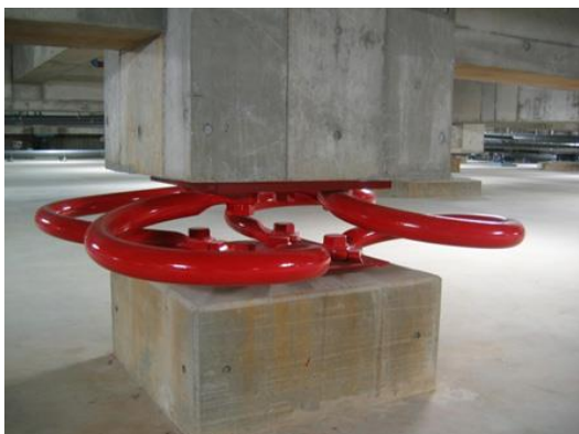
Photo 1: Looped steel-bar damper for seismic isolation
