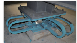
Condition of steel damper after earthquake
